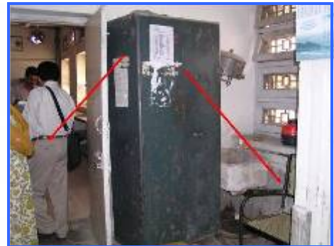
The cupboard is not fixed to the wall, it might fall and block the emergency exit
